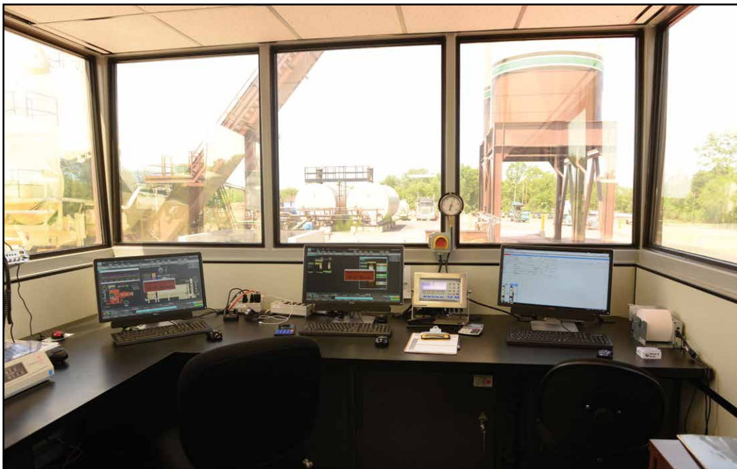
A 10 ft x 30 ft (3.05 m x 9.14 m) power center, complete with a Total Control II-HMA PLC control system, handles operations for the Walsh & Kelly La Porte plant.
