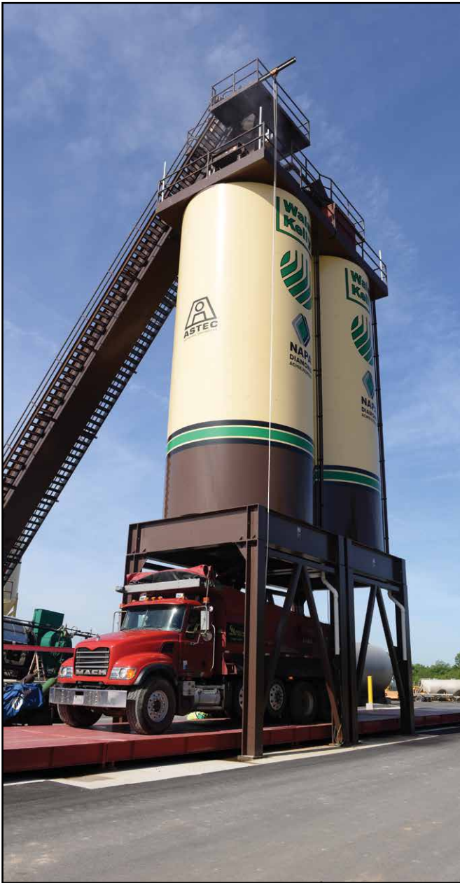
Walsh & Kelly customized the La Porte asphalt facility with two, 200-ton (181 tonne) New Generation Storage System silos.
