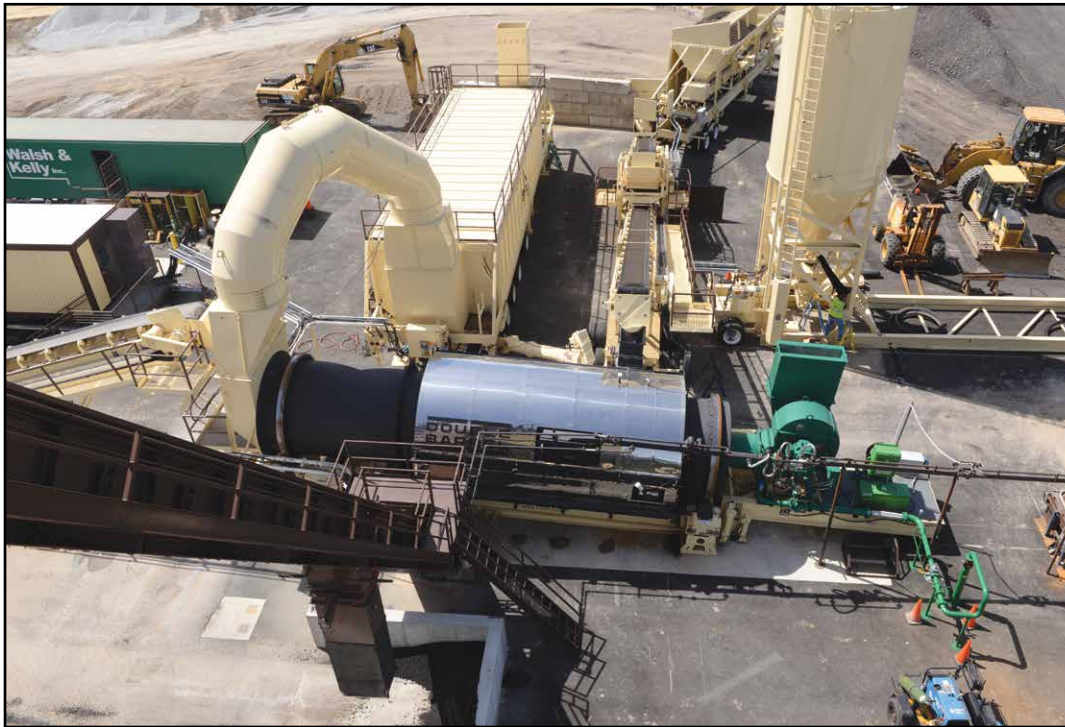
Wash & Kelly's La Porte plant has a portable 8 ft (2.44 m) Double Barrel® drum mixer, a Phoenix® Talon burner, and a portable 66,782 CFM Express Baghouse with inertial dust separator.
